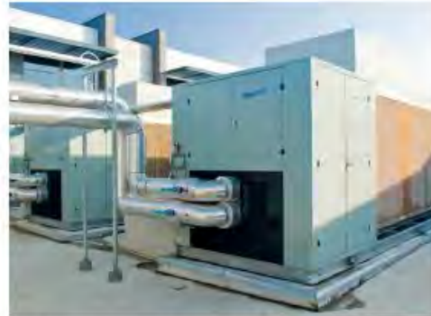
Use of evaporative pre-cooling to minimize air-cooled power consumption can be very efficient from an operating cost perspective.
