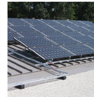
Solar rooftop system generates energy without compromising rooftop performance.
