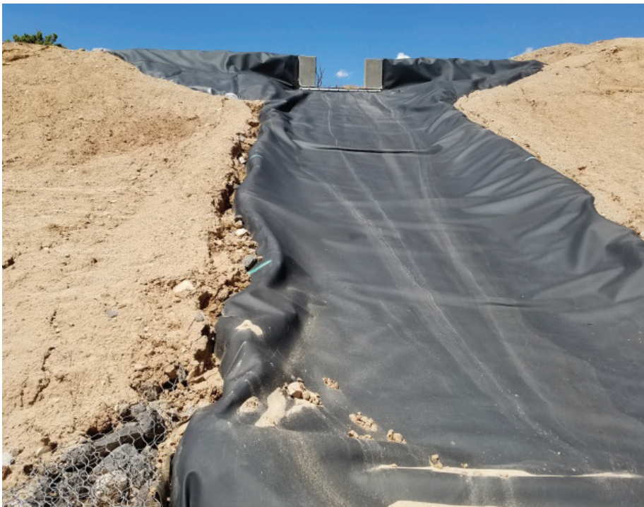
HDPE-lined stormwater diversion channel at a regional landfill facility.
