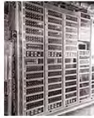
First Domestic-made Automated Switching System in 1956
