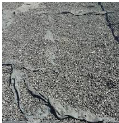
Geotextile fabric should never be exposed and is a sure sign that surfacing levels are inadequate.
