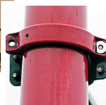
The clamp on this equipment is missing hardware which must be replaced.
