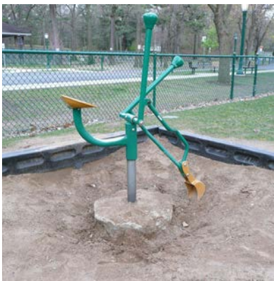
The exposed footer on this equipment is a hazard and should be covered with surfacing.
