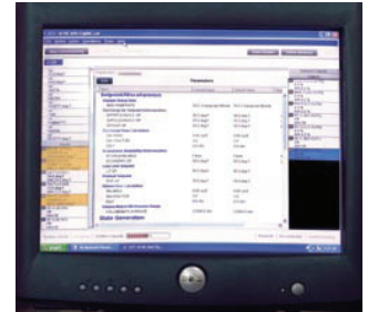
Factory-testing ensures that all controls work appropriately.
