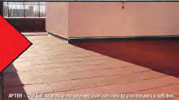
AFTER - Our ballast mats were selected over concrete to give the area a soft feel.
