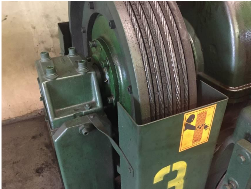
Dirty Hoist Ropes
