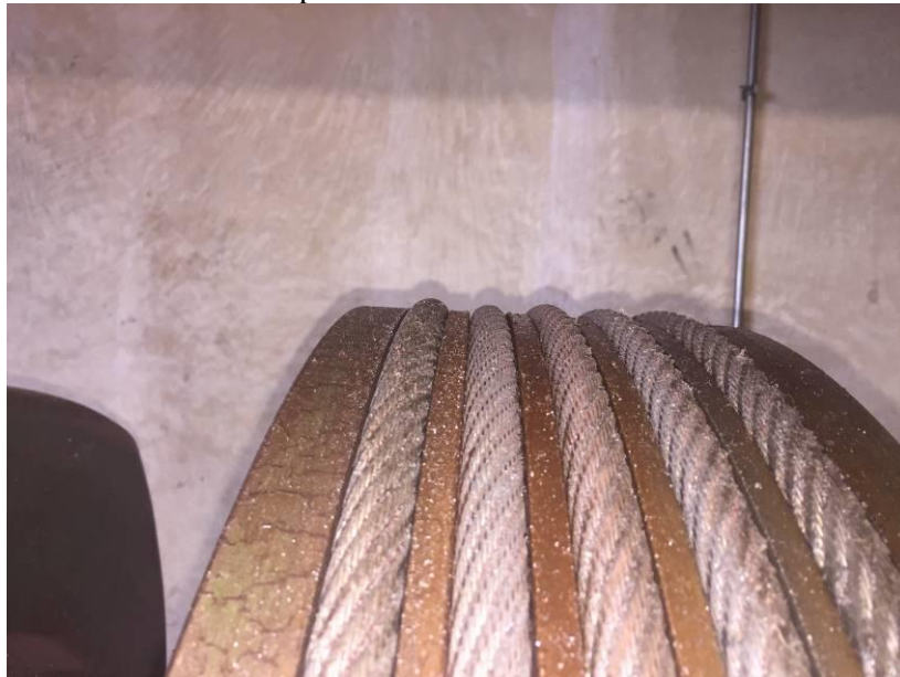
Uneven Ropes in Sheave
