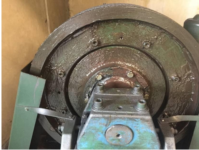
Drive Sheave Seal Failure
