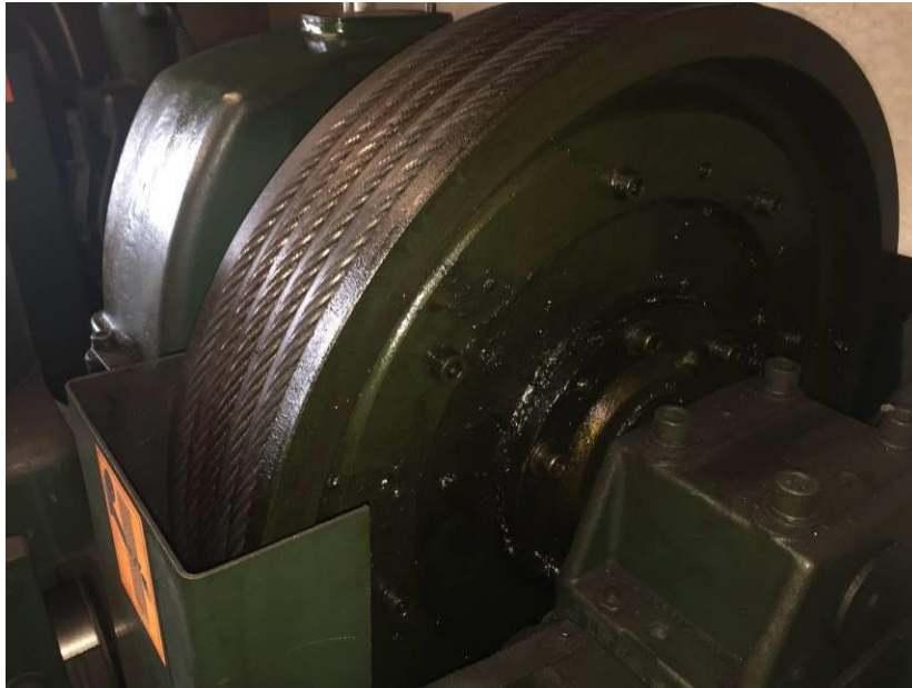
Drive Sheave Seal Failure
