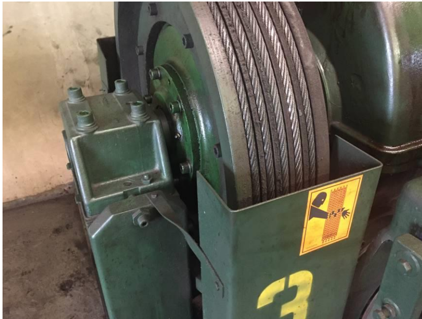
Dirty Hoist Ropes
