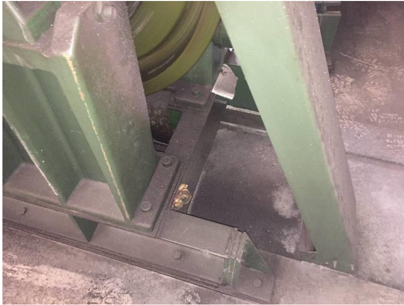
Rope Debris Around Machine
